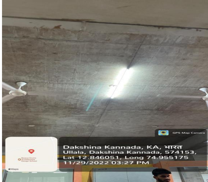
Fig. 3 LED lights in Passage
