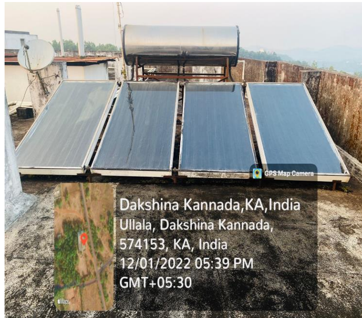
Fig. 8 Solar panels in Staff Quarters
