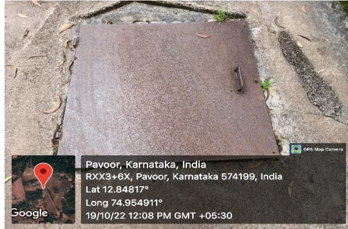
Fig. 8 The sump where water is collected during rainy season
