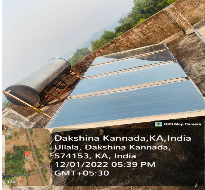
Fig. 7 Solar panels in Staff Quarters
