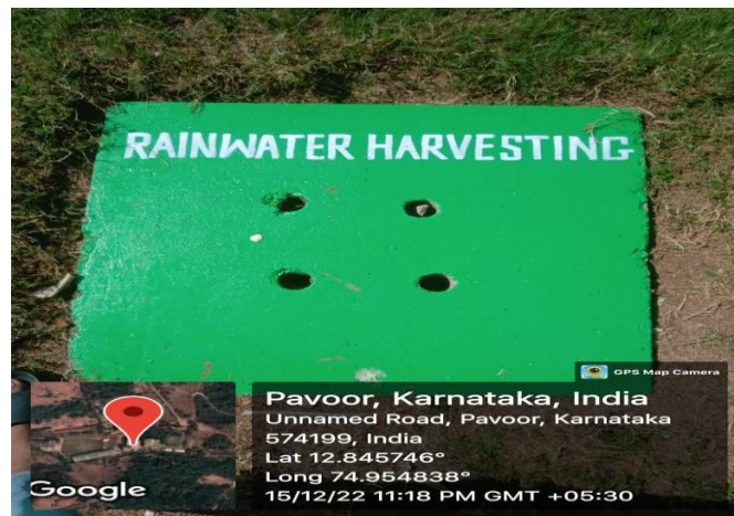
Fig. 2 Recharge well at Location One near Car Parking area
