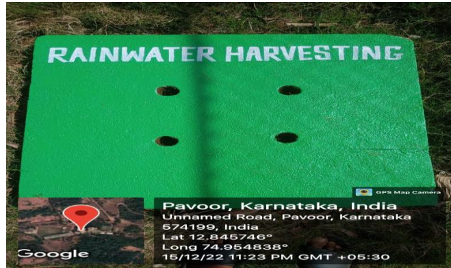
Fig. 6 Recharge well No.5 in the Arena
