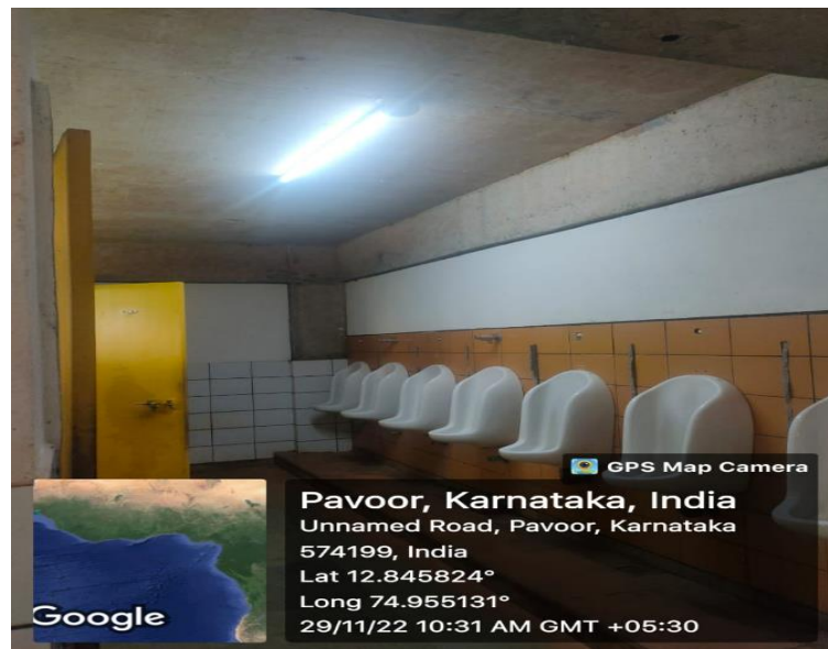
Fig. 2 Energy saving Light sensors in Washroom
